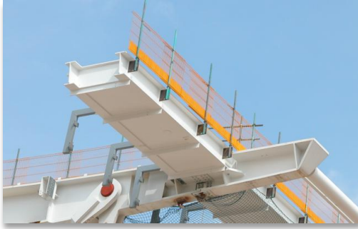
Pre-installed Edge Protection Prior to Lifting
