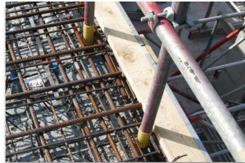
Pre-installed sockets in PC Unit
