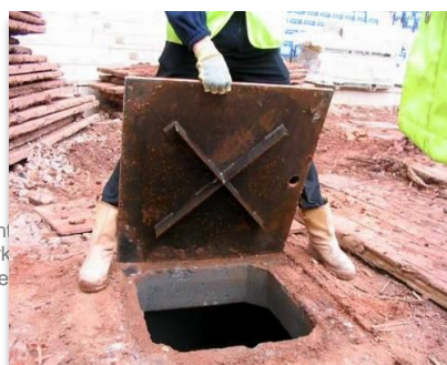
Temporary access chamber cover in trafficked area
